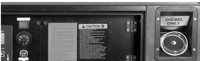
Figure.5A - Diesel fired burner fuel supply tank
