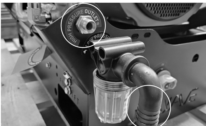
Figure.7 - PMG G2 High Pressure Outlet & Low Pressure Inlet Location
